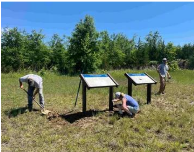
New waysides being installed in Brandy Station Battlefield in Culpeper County, Va. Chuck Laudner
